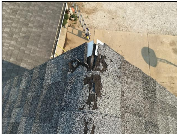
Deteriorated/damaged shingles on dormer ridge
