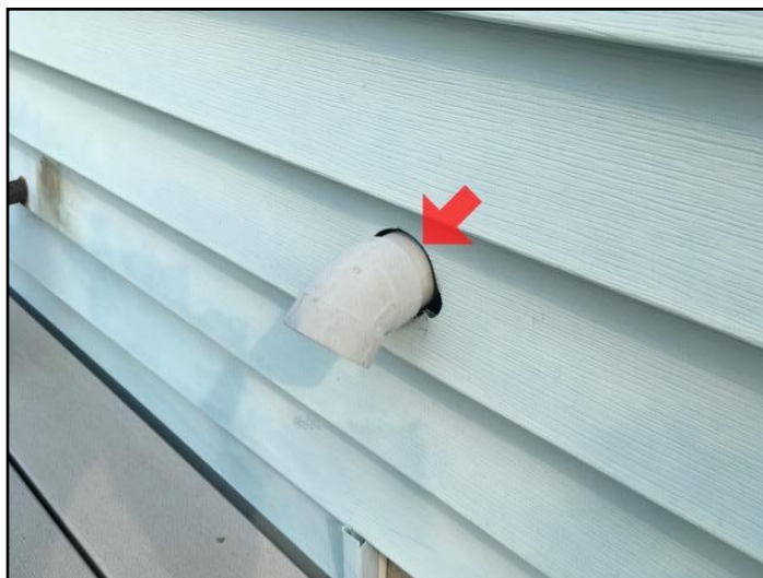
Missing caulk around utility penetration
