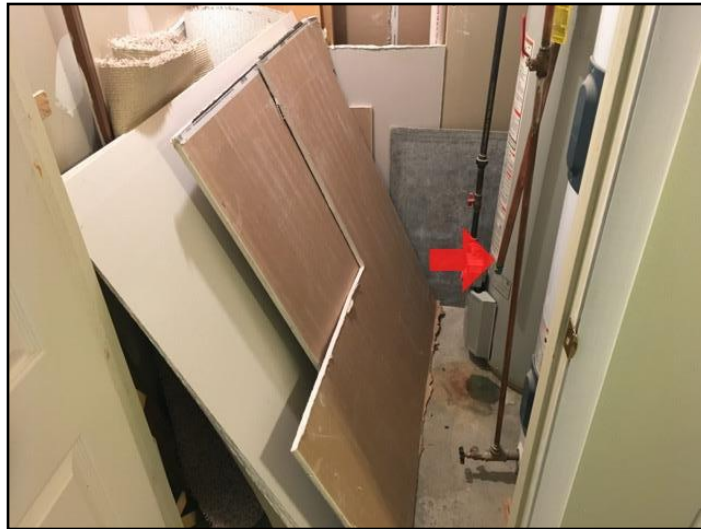
State water heater TPR valve ext. too short
