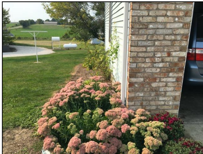
Vegetation/shrubs too close to building
