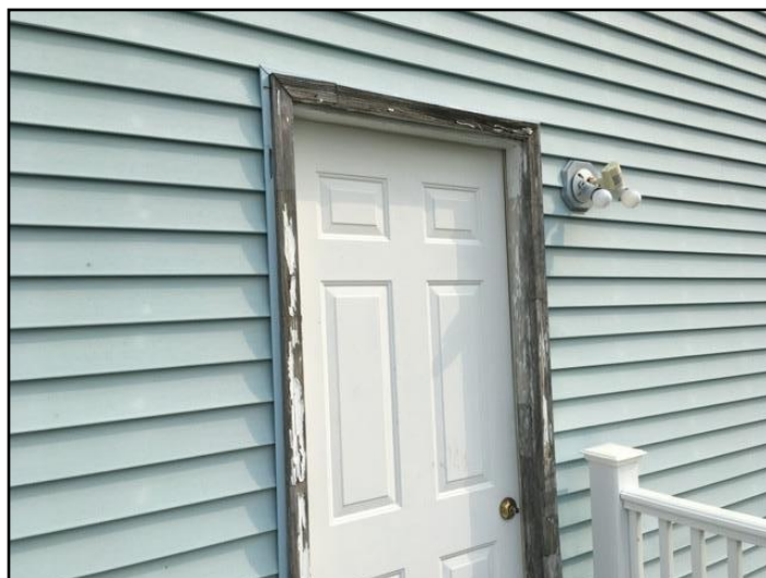
Paint needed on garage service door
