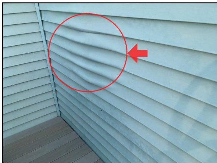
Deformed vinyl siding, from high temp - grill
