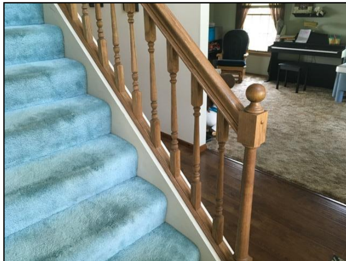
Balusters too far apart
