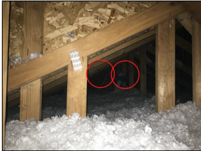
2 bath exhaust fans not vented to exterior
