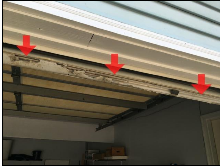
Weatherstripping damaged or missing.
