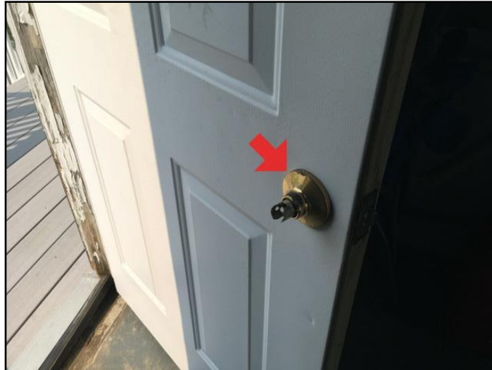
Missing door knob - inoperable from exterior
