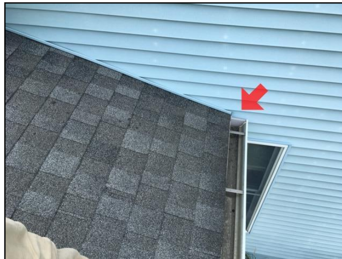
Kickout flashing - missing
