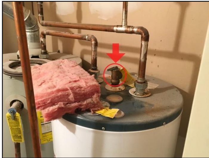
Rheem water heater TPR valve ext. missing
